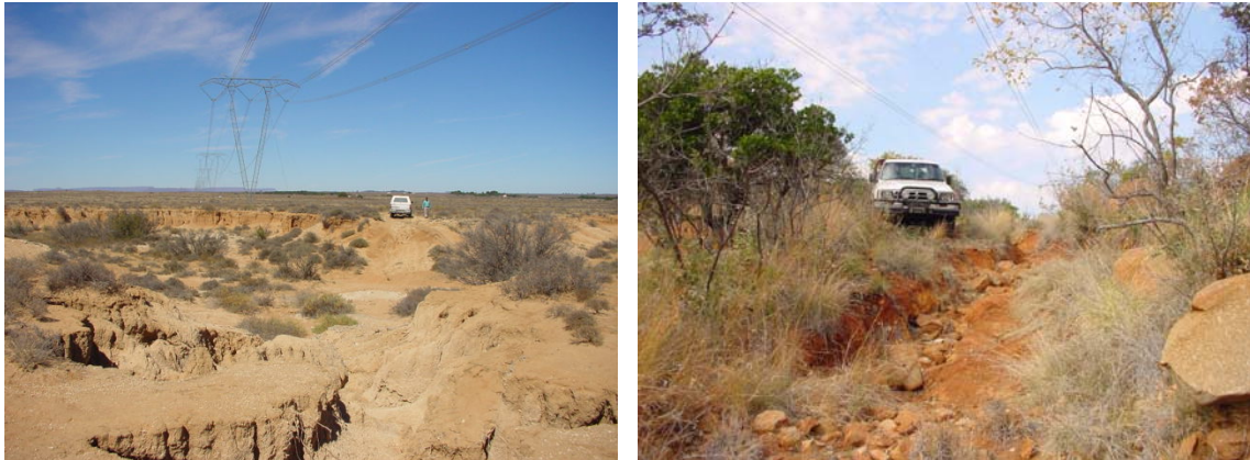
Figure 2. Examples of erosion in the servitude, which hampers access during maintenance and emergencies.
