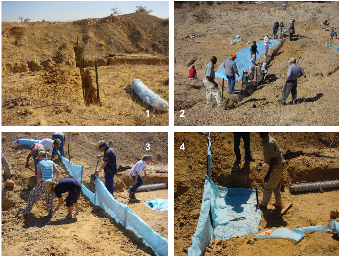
Figure 6 shows the steps in the construction of a silt-screen. Girls from two schools in Pretoria on the Mabula Game farm carried out this exercise. In photo 1 the trench is dug across the erosion channel and Y standards are placed to form the main part of the structure. In photo 2 the Y standards are connected with stay wires and covered with wire mesh. The structure is then covered with a biodegradable geo-textile in photo 3. In photo 4 the structure is completed by adding an apron, made of geo-textile and wire mesh.
