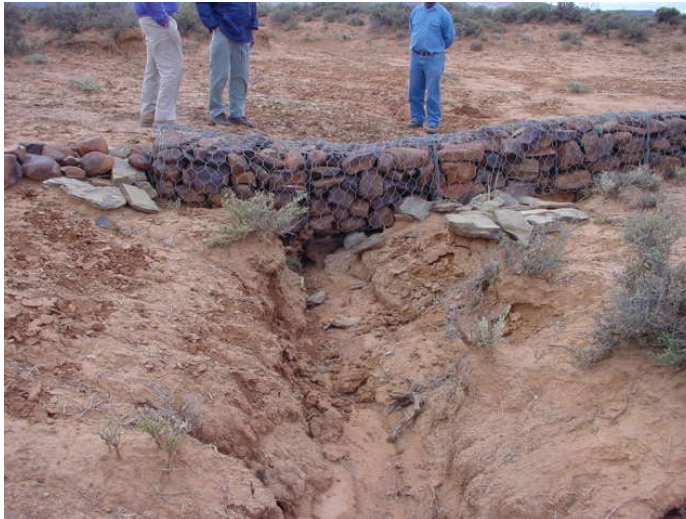
Figure 5. An example of an inappropriately designed gabion. No geotextile or apron was used in this case and erosion eventually occurred under the structure. No provision was made to prevent erosion at the overflow.
